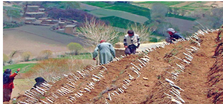
LEFT AND ABOVE | Workers reshaped moderate slopes into contour bunds and planted poplar cuttings during early spring while soils were moist from snow melt. The resulting thickets helped stabilize snowfields and could be thinned for firewood and animal fodder or eventually converted to woodlots. This approach combined slope stabilization with forestry
